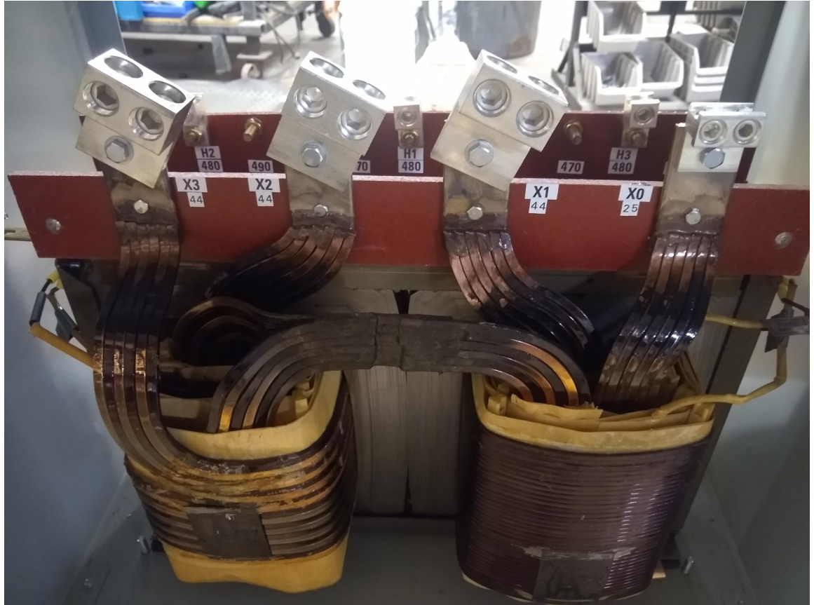
Transformer Primary (Back) and Secondary (Front) Connections
